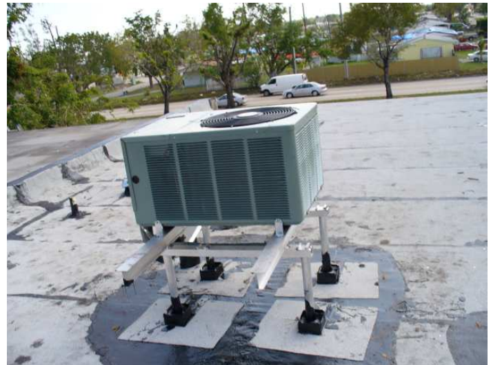
The Clients a/c condensing unit.
