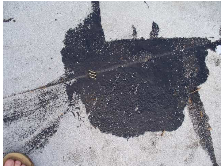
Nails in tar on roof.
