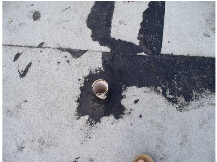
One of the Clients vent stacks.
