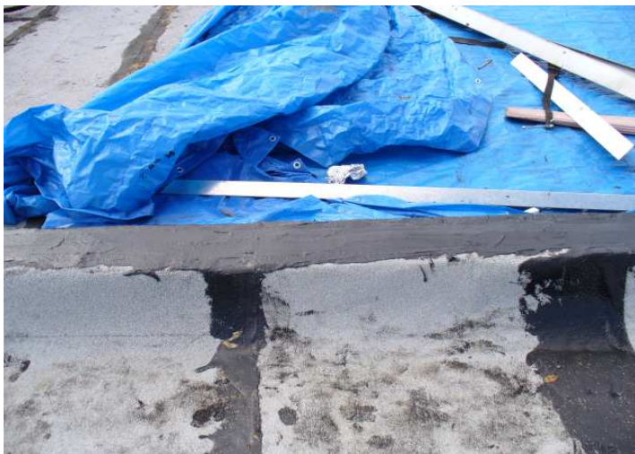
Tar on the roof covering. The entire roof looks like this.
