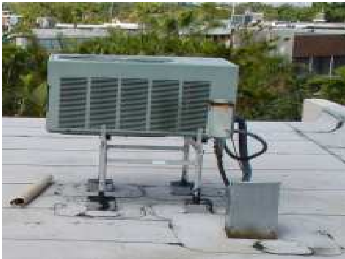
A properly installed a/c condensing unit on the neighbors roof.
