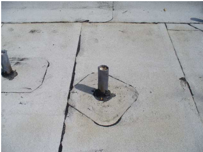
A properly installed vent stack on the neighbors roof.
