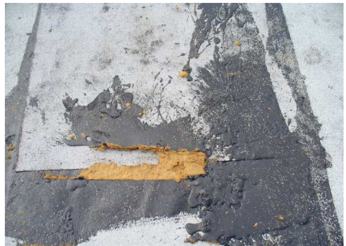
Debris and more tar.
