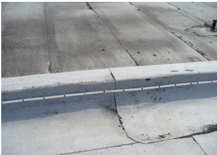
The proper way to secure the ends of the roof to a wall.
