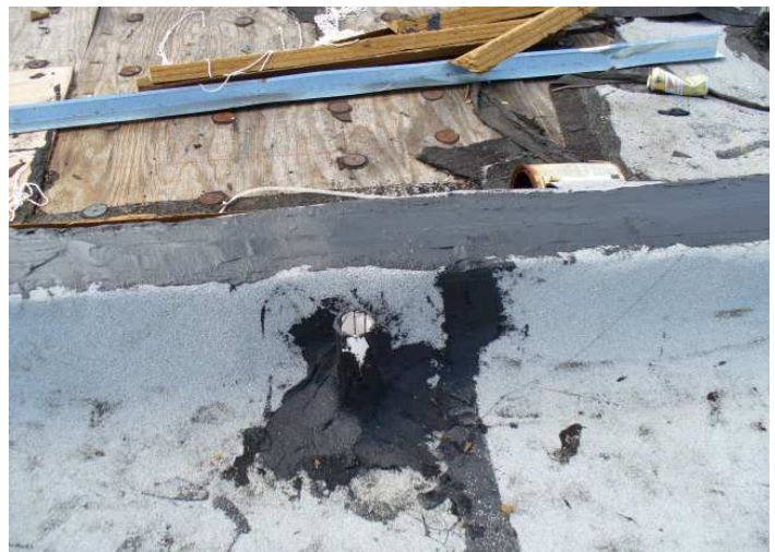
Vent stack number 3 which is very close to the separation wall.
