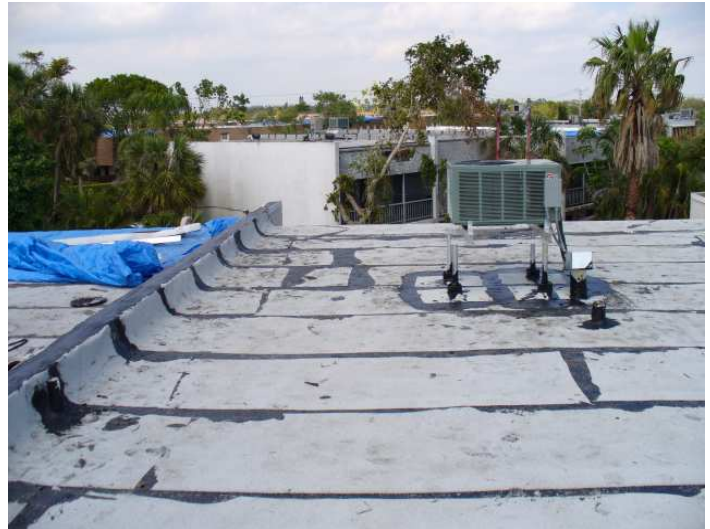
This is the Clients roof. Not completed n a workman like manner.
