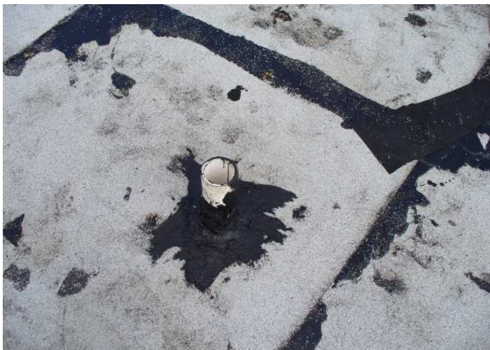
Vent stack number 2.
