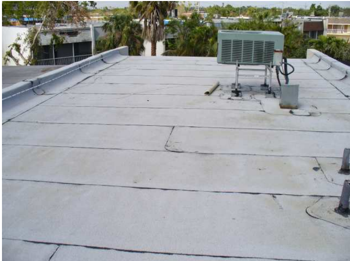
This is the neighbors roof. It has been installed in a professional and workman like manner.
