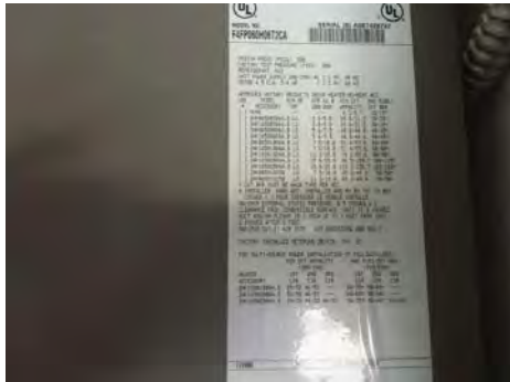
Air handler data plate.
