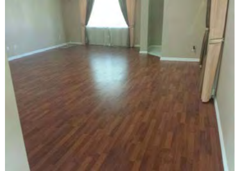
Flooring at front living room was damaged (cupping usually caused by improper installation methods).
