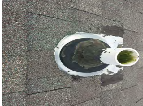
One vent stack boot was torn at the second story roof.
