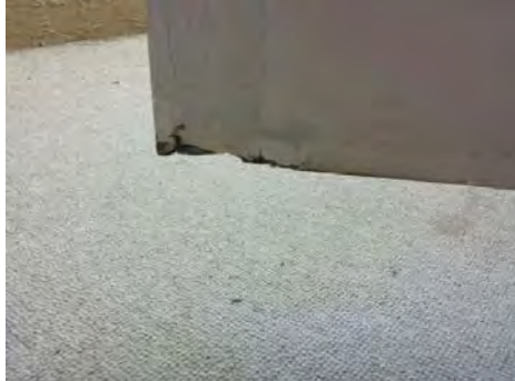
Front door was rusted out.
