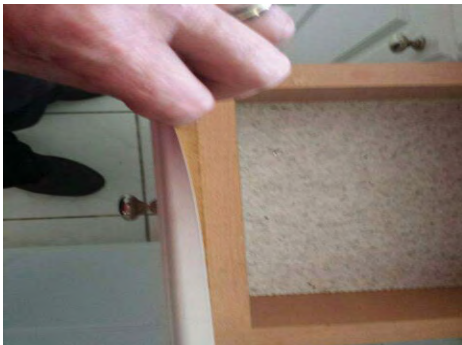
The covering was peeling off of several kitchen cabinet doors and drawers.
