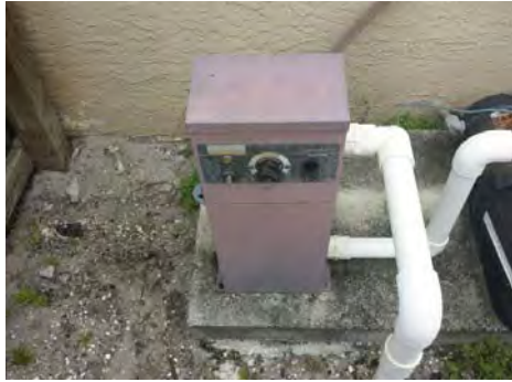
The pool heater was not operating long enough to test properly. Re-test prior to purchase.
