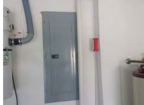
Central vacuum line was routed in front of the distribution panel in the garage.
