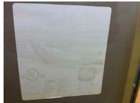
Condensing unit data plate.
