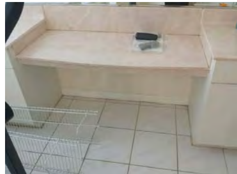
The shelf between the two sinks in the master bathroom was warped/damaged.
