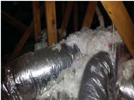
Duct work in attic.
