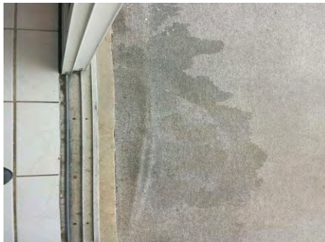
Dishwasher was leaking during operation.
