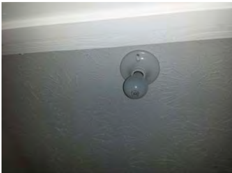
Improper light fixture observed in downstairs closet. No globe was present and damage to the bulb may result.
