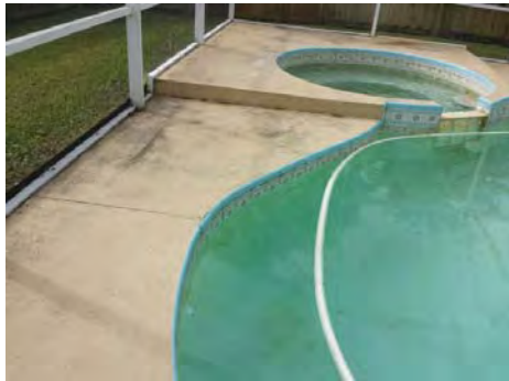
Several pool tiles were cracked and loose around the pool.
