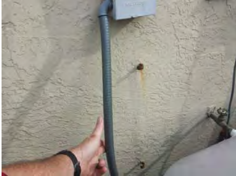
Conduit for a/c condensing unit was not secured.
