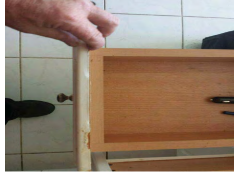
The covering was peeling off of several kitchen cabinet doors and drawers.
