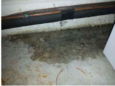
Washing machine was leaking during operation.
