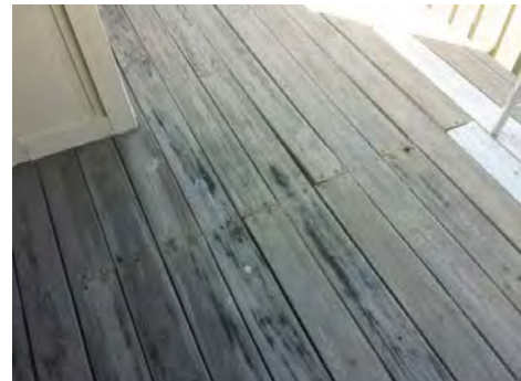
Various areas of damaged railing and decking observed at front balcony.
