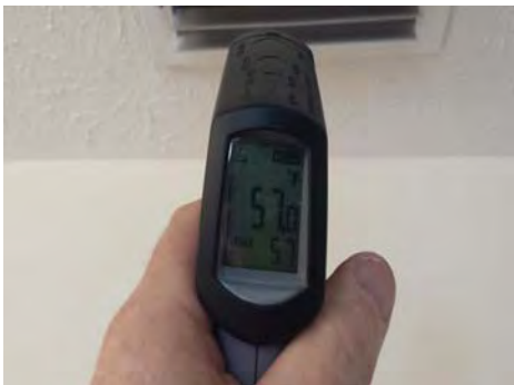
Cooling cycle being tested.
