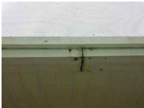
Rear patio gutter was leaking.
