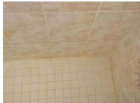
There were several loose tiles observed at the master bathroom shower.
