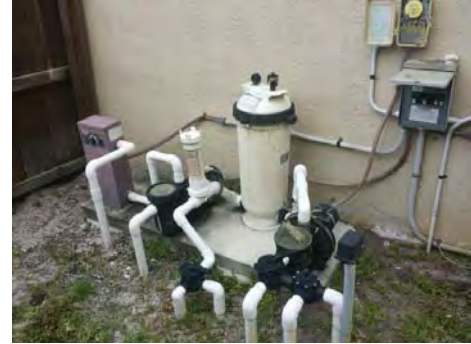
Pool equipment at right rear corner of house.
