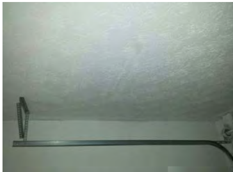
Damaged ceiling observed in garage under balcony.
