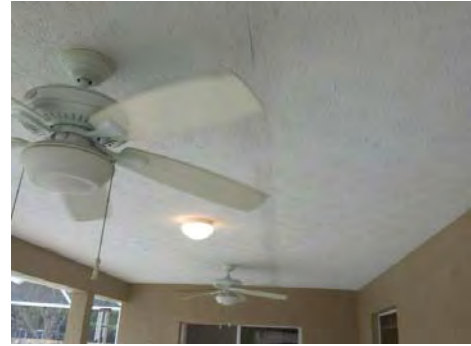
Damage observed at several areas of rear patio ceiling.
