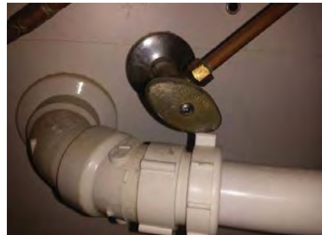
The shut off valve for the left side master bathroom sink was installed in a manner which prevents the valve from being used. It makes contact with the drain line.
