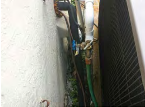
The main water shut off and hose bib were directly in back of the a/c condensing unit.
