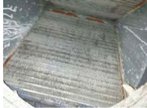
Coils were dirty restricting air flow at air handler.
