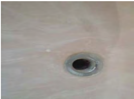
Drain stopper was not present at master bathroom right side sink.
