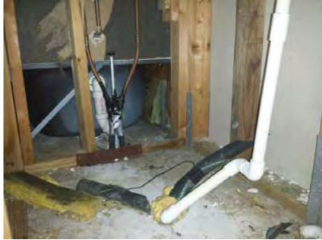
Intake was damaged/unfinished at air handler.
