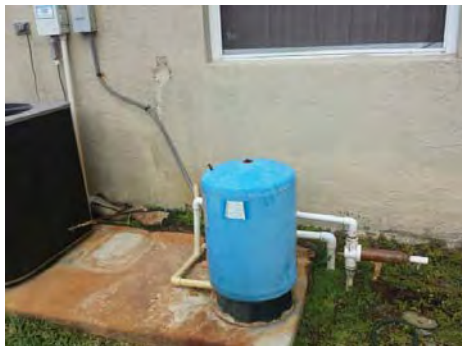
Sprinkler equipment at right side of house.
