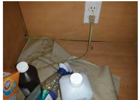
Kitchen sink base cabinet was damaged, possibly from current water leak or dishwasher leak.
