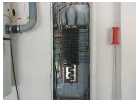
Distribution panel in garage with cover removed.
