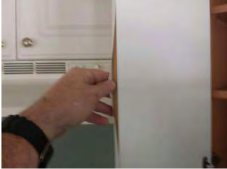
The covering was peeling off of several kitchen cabinet doors and drawers.
