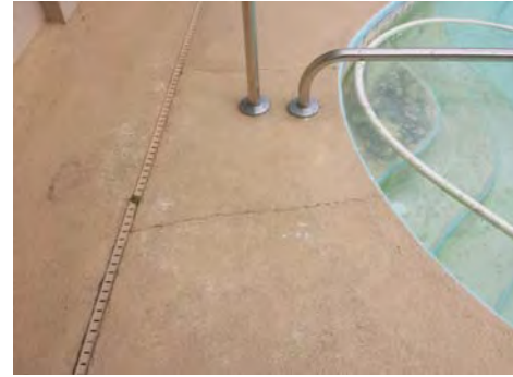
There were several cracks in the patio deck that were entering the pool.
