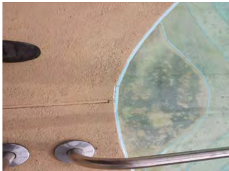
There were several cracks in the patio deck that were entering the pool.
