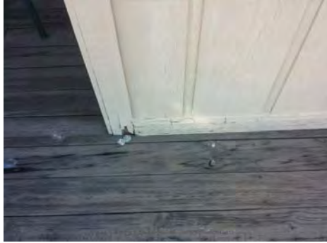
Various areas of damaged siding and trim observed at front balcony.
