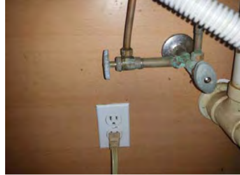
Leak observed at hot side of kitchen sink faucet.
