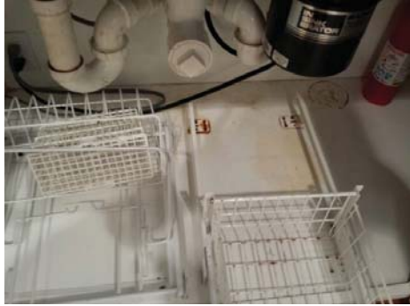
Minor damage observed at kitchen sink base cabinet shelf.
