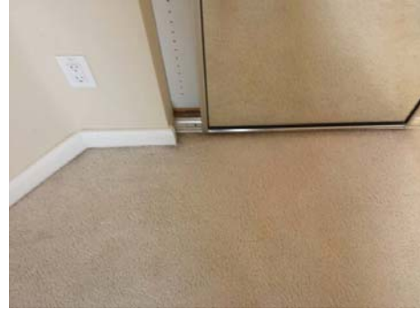
Upstairs bedroom closet doors require adjustment and possibly a new lower guide at the master bedroom.
