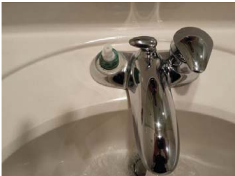
Hot water handle was broken at the upstairs hall bathroom sink and was leaking as well.
