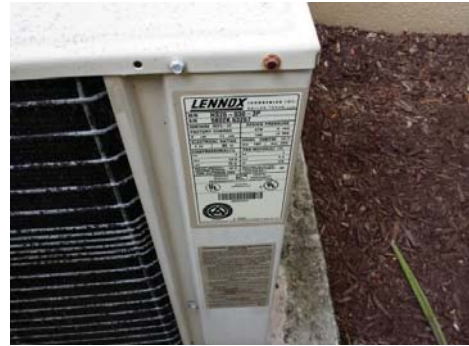
Condensing unit data plate.
