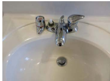
Hot water handle was broken at both sinks in master bathroom. The right side sink handle was also leaking.
