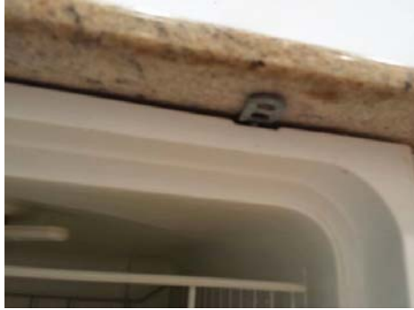
Dishwasher was not mounted properly.
