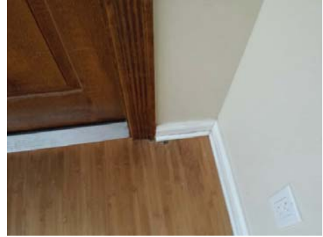
Damaged frame and door observed at rear living room leading to the patio.
