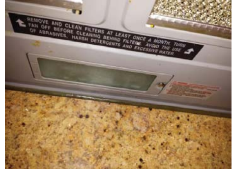
Bulb did not function at hood fan.
