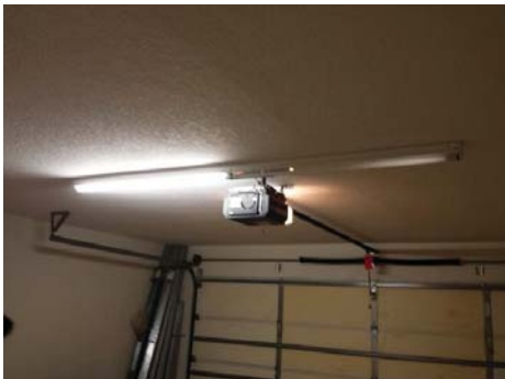
Cover was not present at garage lights and damage to bulbs may result.
