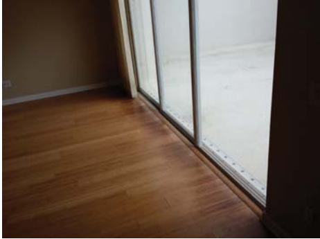
Damaged flooring observed at rear of living room leading to the patio.
