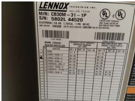
Air handler data plate.
