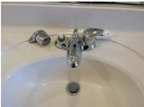
Hot water handle was broken at both sinks in master bathroom. The right side sink handle was also leaking.
