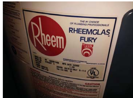
Water heater data plate.
