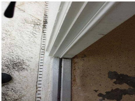
Damaged door frame observed at garage pedestrian entrance door.
