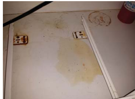
Kitchen faucet was very difficult to move and also was leaking.
