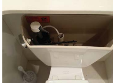
The toilet in the upstairs hall bathroom did not fill (ball/cock assembly).
