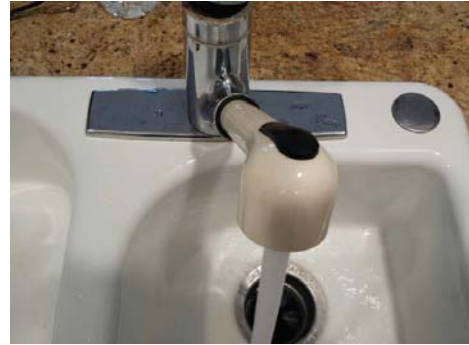
Hand sprayer did not function at kitchen faucet.
