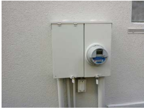
Main service disconnect at left side of house
