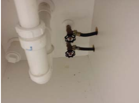
The shut off valves for the washing machine were located under the laundry room sink, and stacked on top of each other. The hot is required to be on the left side, when facing the fixture.
