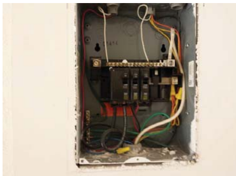
Distribution panel in garage with cover removed.
