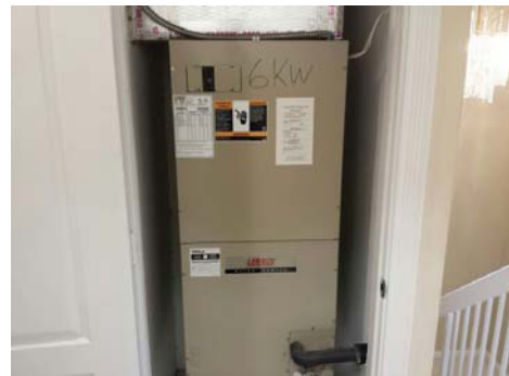
Air handler in upstairs hall closet.
