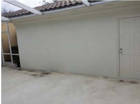
Water was collecting in several areas of the rear patio.
