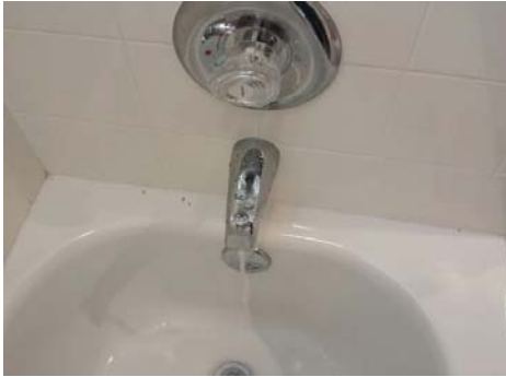
There was no water pressure present at the hot side of the downstairs bathroom tub/shower.
