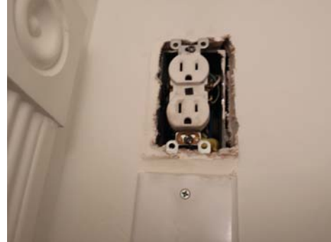
Faceplate was not secured at receptacle under staircase.
