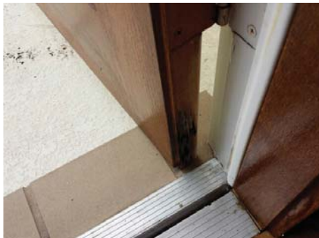
Damaged frame and door observed at rear living room leading to the patio.
