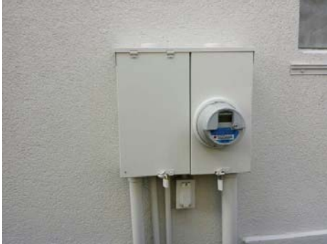
Lock was present on main service disconnect panel. (Remove)
