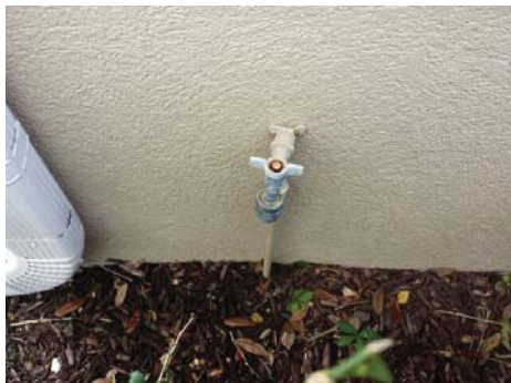
Main water shut off at right side of garage.
