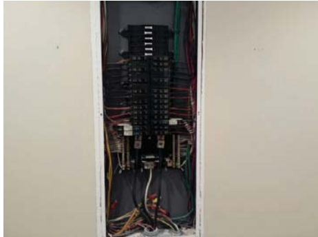
Distribution panel in kitchen with cover removed.
