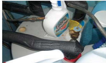
Water heater top
