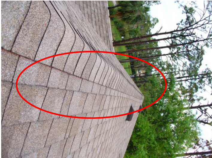
Uneven row of shingles on front of roof.
