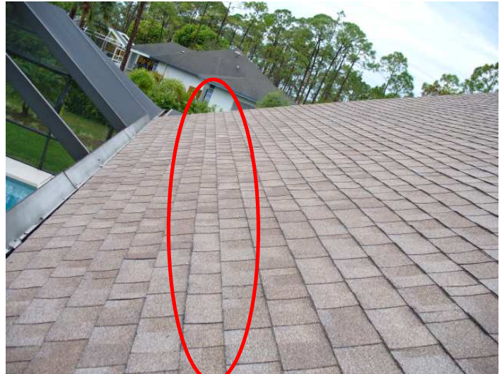
Uneven row of shingles on rear of roof
