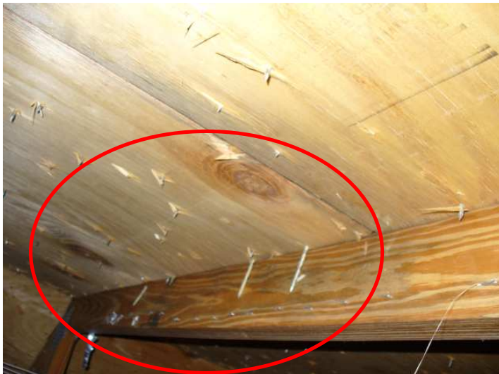
During the re-nailing of the plywood, several nails missed the truss.
