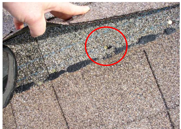
Nail over-driven through shingle. There were several nails over driven throughout the roof.
