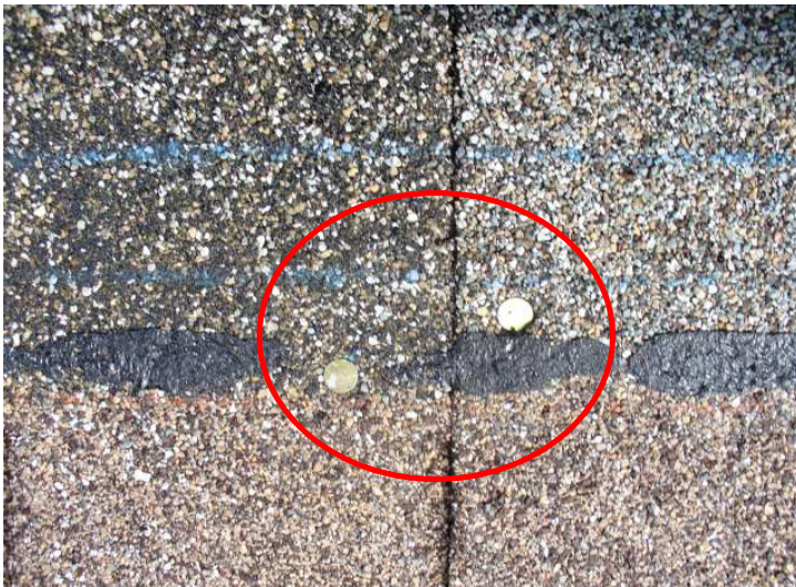
One nail too low, the other nail not nailed in far enough. There were several shingles installed in this manner.
