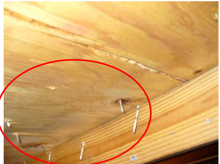
More missed trusses.
