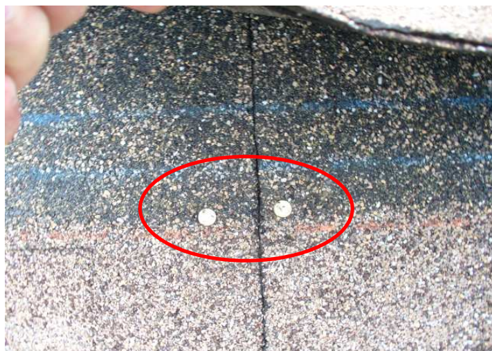
Nail too close to the edge of the shingle (1-1/2 inch required).
