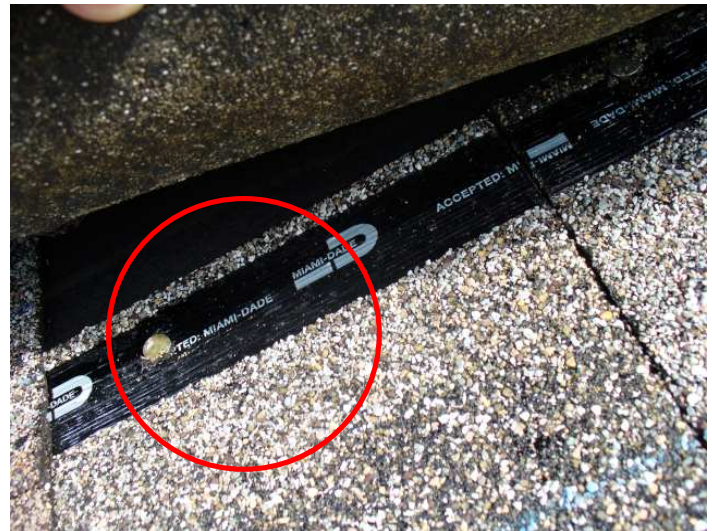
Nail in the rear strip. Several were like this as well.
