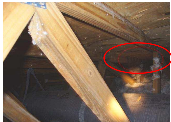
There are six nails that missed the truss in a 2 foot span. There were over 400 nails like this.
