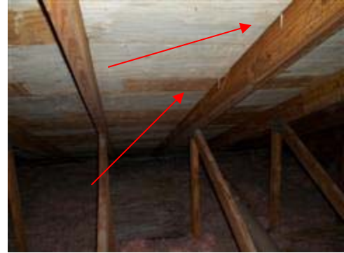
Several nails that missed the trusses were still present on mostly, the front portion of the roof.
