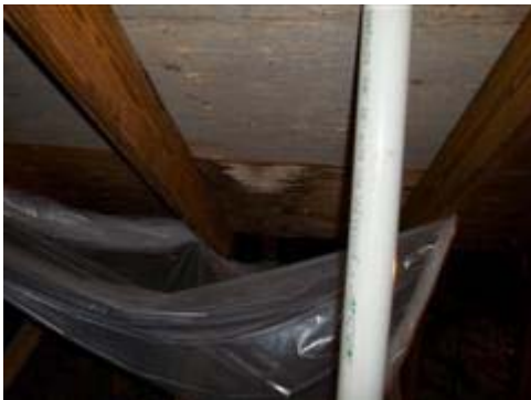
Damaged decking observed from what appears to be a roof leak at the garage vent stack.
