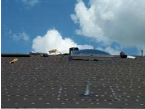
The tar paper has been cut in numerous areas in order to facilitate removal of the nails that missed the trusses.
