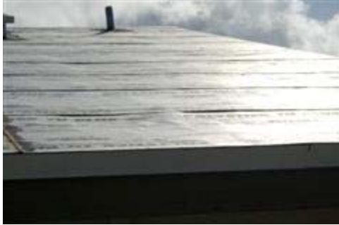
Membrane not adhered properly.
