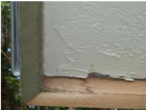
Evidence leak observed at right side front fascia.
