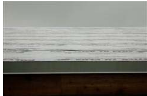
Membrane not adhered properly.
