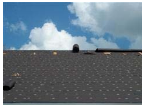
The tar paper has been cut in numerous areas in order to facilitate removal of the nails that missed the trusses.
