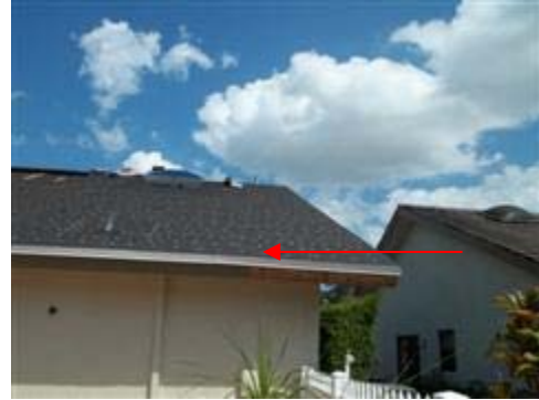
Left rear side off roof decking was sloped over the edge of the support wall.
