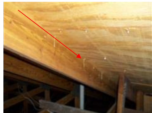
Several nails that missed the trusses were still present on mostly, the front portion of the roof.
