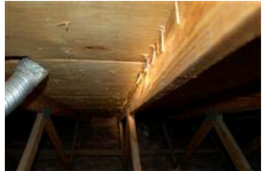
Hole for vent bathroom vent fan line should be enlarged to accommodate the two other bathroom vent fan lines.
