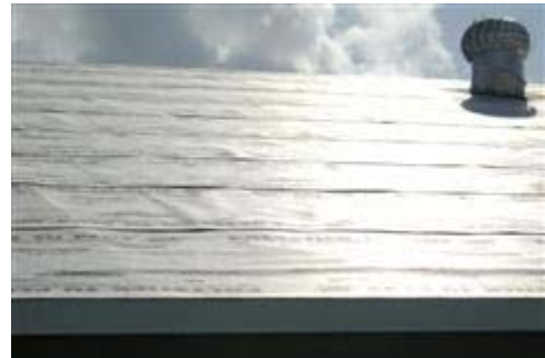
Membrane not adhered properly.
