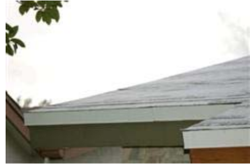
Membrane not adhered properly.
