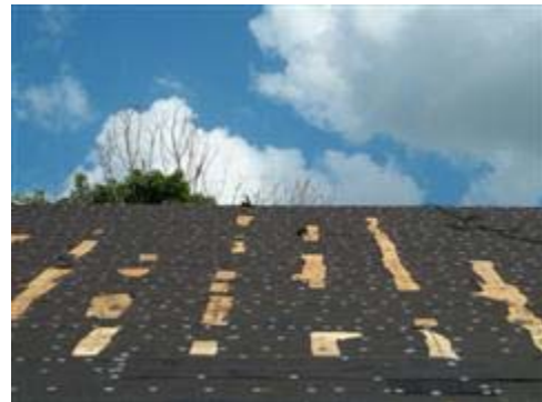
The tar paper has been cut in numerous areas in order to facilitate removal of the nails that missed the trusses.
