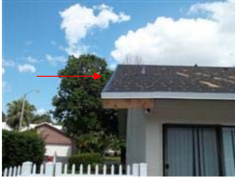
Right rear side off roof decking was sloped over the edge of the support wall.
