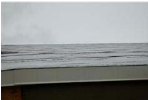
Membrane not adhered properly.
