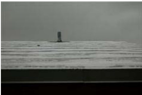
Membrane not adhered properly.
