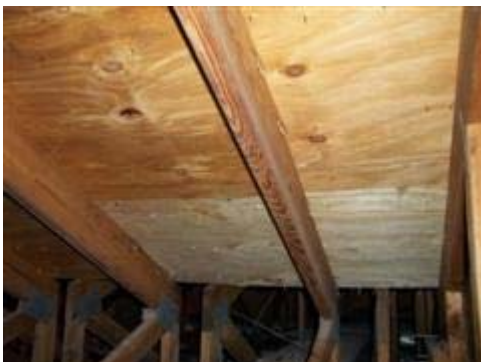
Debris scattered in various areas of the attic as well as on the a/c duct work.
