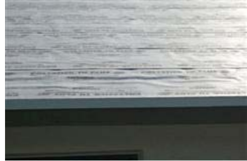
Membrane not adhered properly.
