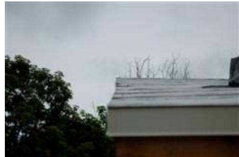
Membrane not adhered properly.
