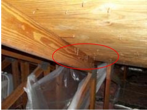
Several nails that missed the trusses were still present on mostly, the front portion of the roof.
