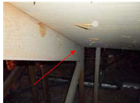
Several nails that missed the trusses were still present on mostly, the front portion of the roof.
