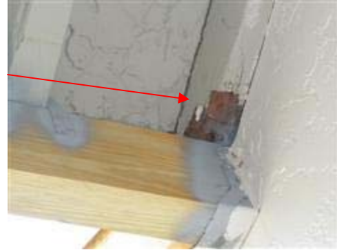
Damaged beam observed at front porch.
