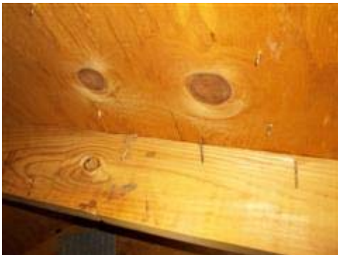
Several nails that missed the trusses were still present on mostly, the front portion of the roof.
