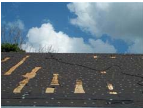
The tar paper has been cut in numerous areas in order to facilitate removal of the nails that missed the trusses.
