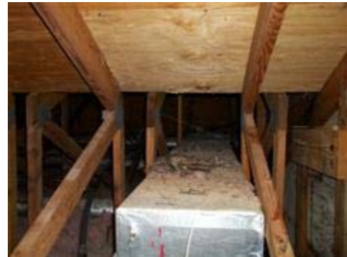
Debris scattered in various areas of the attic as well as on the a/c duct work.
