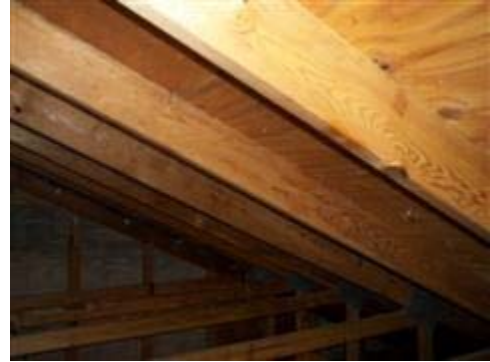
Several nails that missed the trusses were still present on mostly, the front portion of the roof.
