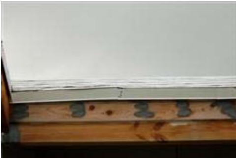
Membrane not adhered properly.
