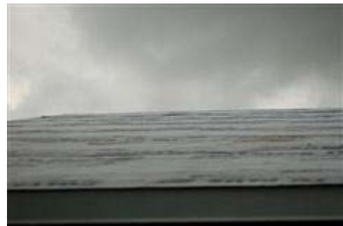
Membrane not adhered properly.
