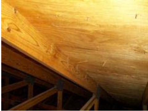
Several nails that missed the trusses were still present on mostly, the front portion of the roof.
