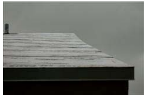
Membrane not adhered properly.
