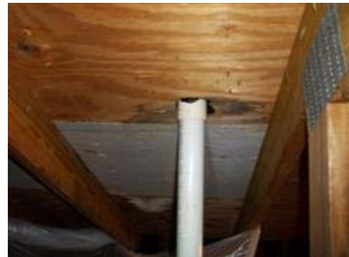
Damaged decking observed from what appears to be a roof leak at the garage vent stack.
