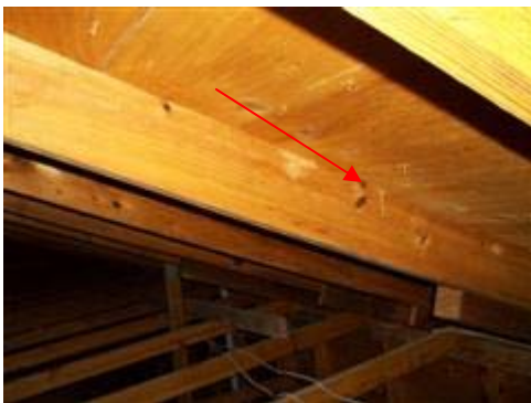
Several nails that missed the trusses were still present on mostly, the front portion of the roof.
