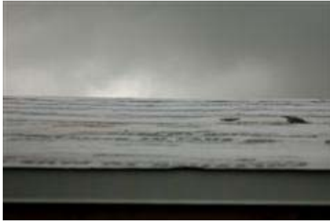
Membrane not adhered properly.
