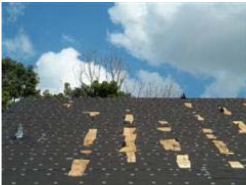
The tar paper has been cut in numerous areas in order to facilitate removal of the nails that missed the trusses.
