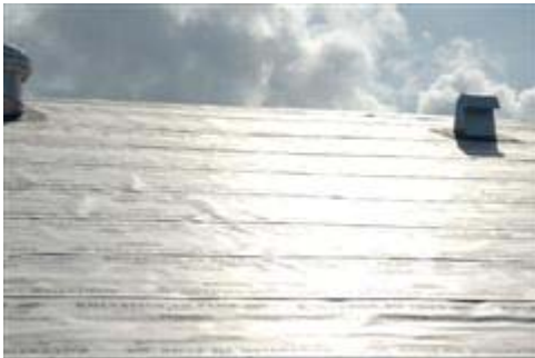
Membrane not adhered properly.
