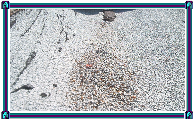
Dip in front flat roof where water has collected.
