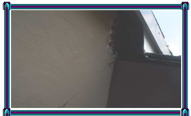
Void at left side of front porch.
