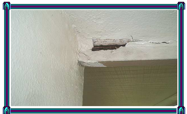
Damaged fascia at front entrance.
