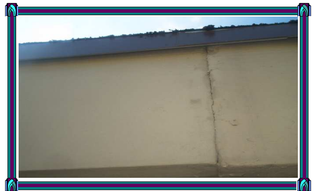
No drip edge at rear of house.
