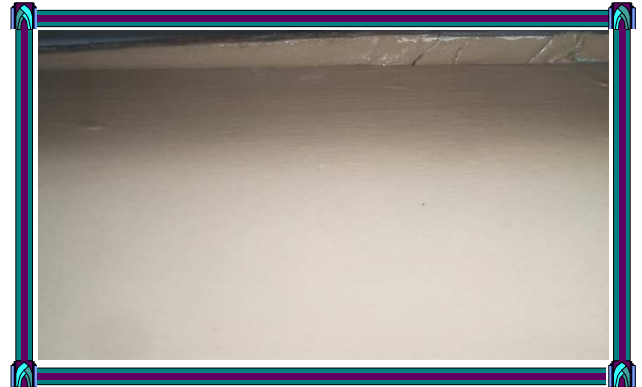
Missing drip edge at left front of house.
