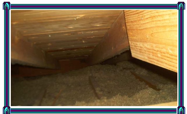
Beam that is not secured to the support wall.
