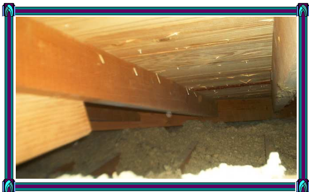
More nails missed the beam.
