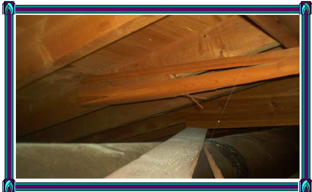
Broken support at another beam that was not secured to the support wall.
