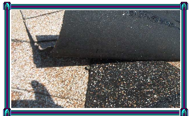
Nail missed shingle.
