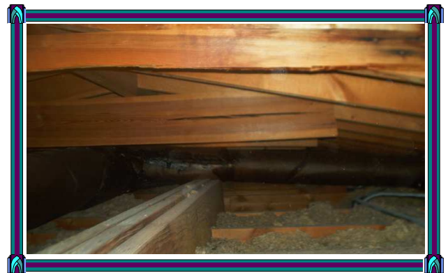
Broken support at center of attic on beam that is not secured to the support wall.
