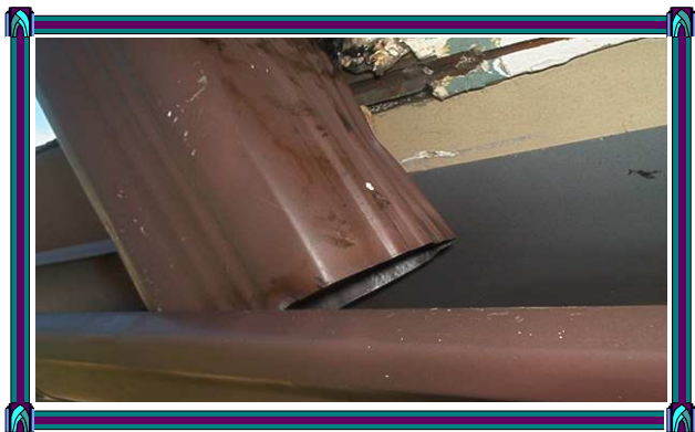
Improperly flashed sheathing at right front entrance porch.
