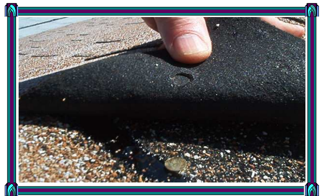
Nail not driven deep enough.
