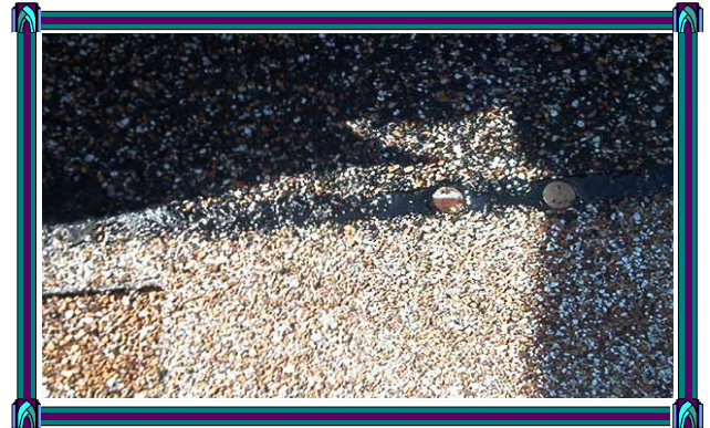
Nails in the center of the shingles are not spaced apart.
