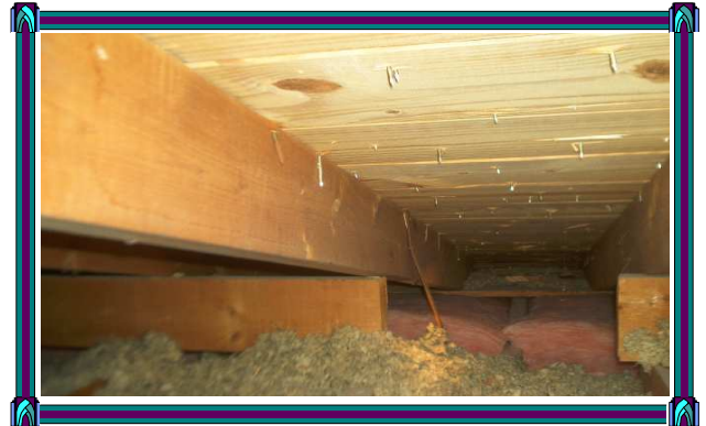
Numerous nails that have missed the beams.
