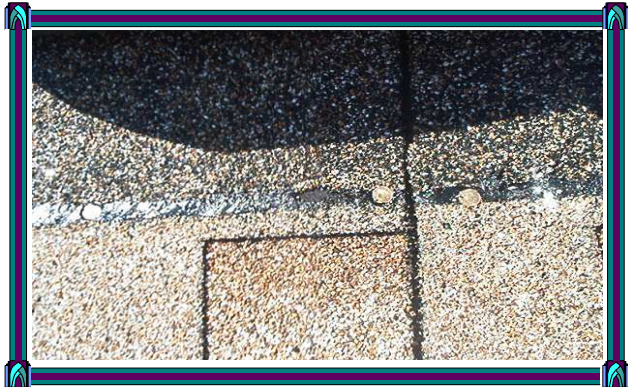
Shingles nailed improperly. Nails are required to be at least 1 1/2 inches from the edge.
