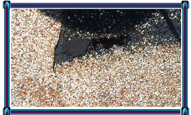
Shingles not nailed down.
