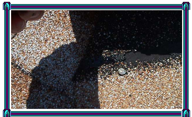
Nail not driven deep enough and shingle is sticking up.
