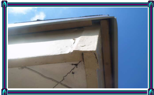
Missing drip edge and rotted fascia at rear of house.
