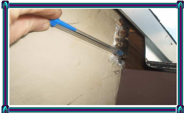
Void at left side of front porch.
