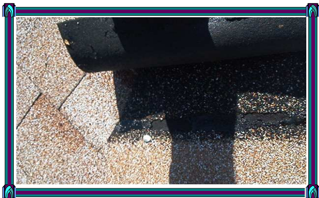
Shingles nailed in tar strip.
