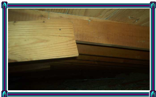
Nails that have missed the beam.
