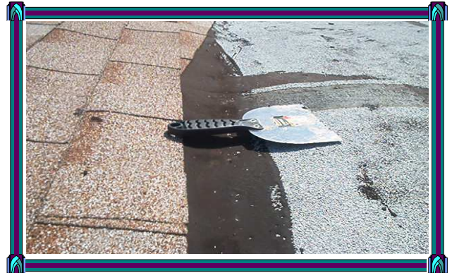
Hump in front flat roof which has cause a valley to form and water ends up in the previous dip.
