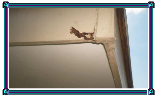
Rotted fascia at left side eof house.
