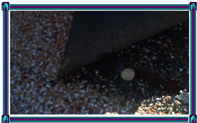
Nail not driven deep enough.
