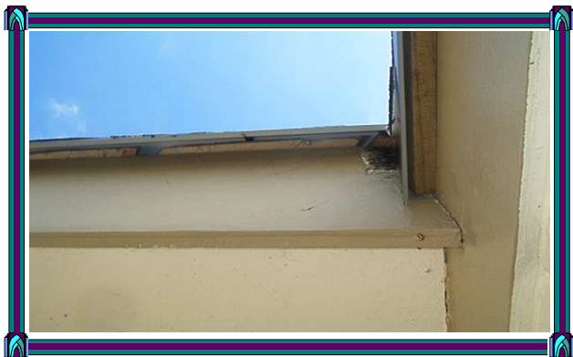
Missing drip edge and void at left front of porch.
