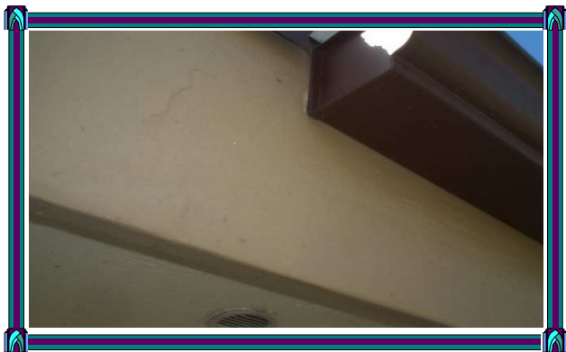
Damaged flashing at rear of house due to gutter installation.
