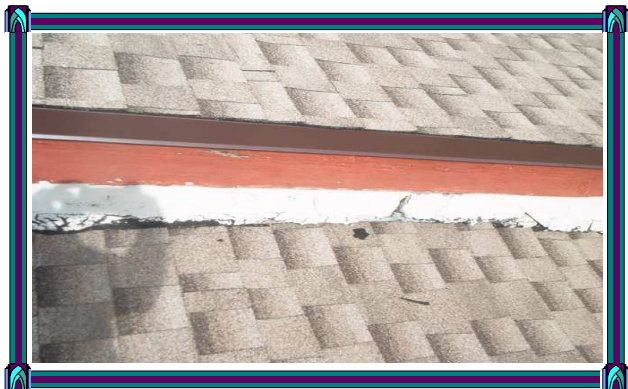
Damaged stucco at roof flashing. The homeowner stated water was entering at this point. Due to the numerous voids, water is most likely entering the structure.
