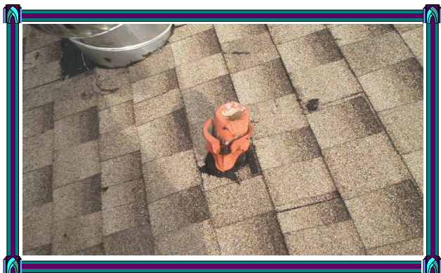
Vent stack sleeve that was not changed.
