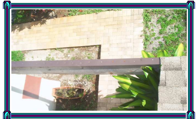
Metal flashing nailed from above at decorative beam. The nails have already started to rust. The beam will rot prematurely.
