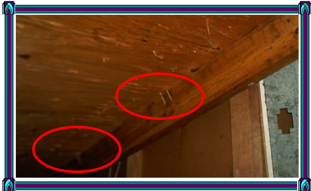
More nails that missed the trusses.
