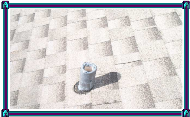
Another vent stack that was not changed.
