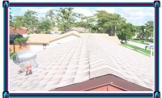
Uneven shingle installation at peak of roof.
