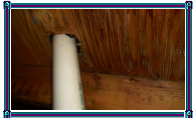
Rotted/damaged decking observed at right side vent stack.
