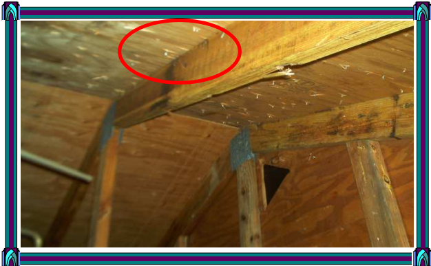
Nails that have missed the trusses. There were a few nails like this throughout the roof.
