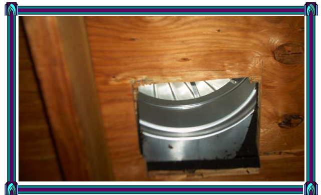
The right side turbine fan is installed in a manner that only allows for a third of the fan to be used.
