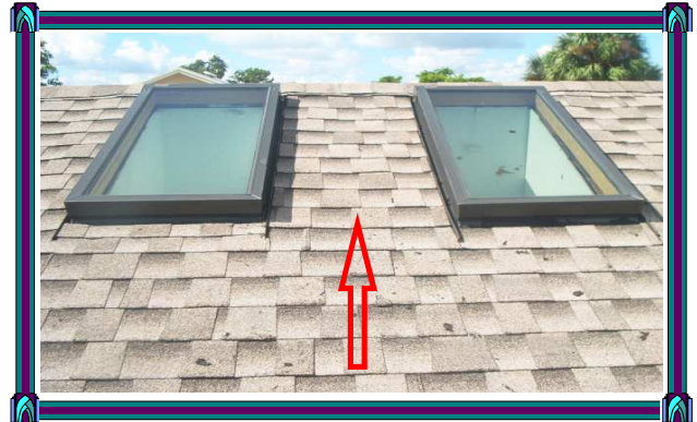
Dip in plywood decking between skylights.
