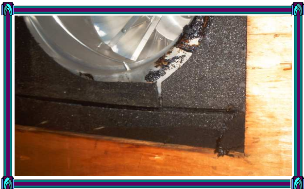
Missing plywood observed at left side turbine fan. There is no wood under the metal lip of this turbine fan base.
