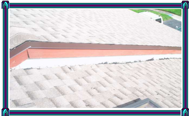
Full view of damaged stucco and exposed wire mesh at living room/garage roof joint.
