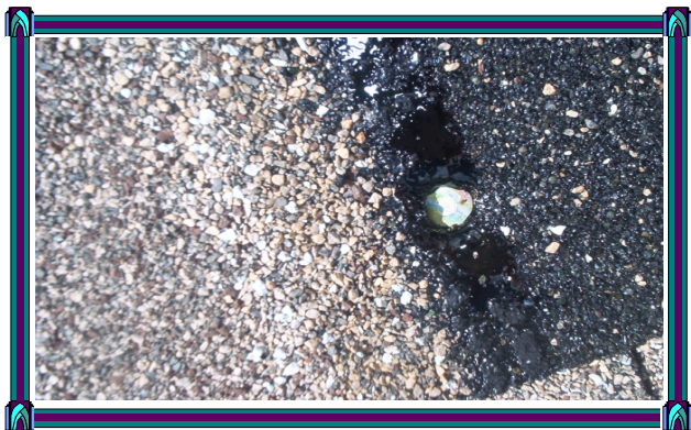
Over-driven nail at center of roof.
