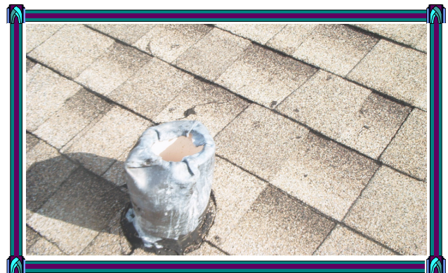
Another vent stack that was not changed.
