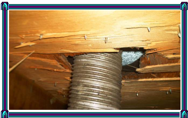
Rotted/damaged decking at dryer vent stack.
