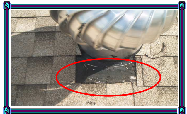
This is the base of the turbine fan. There is no wood under the metal flap.
