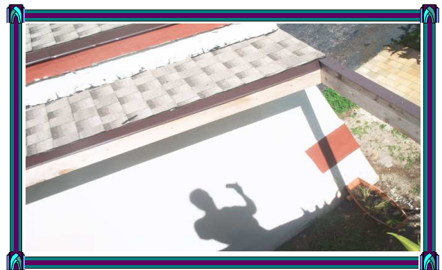
More damaged stucco at living room/garage roof joint.
