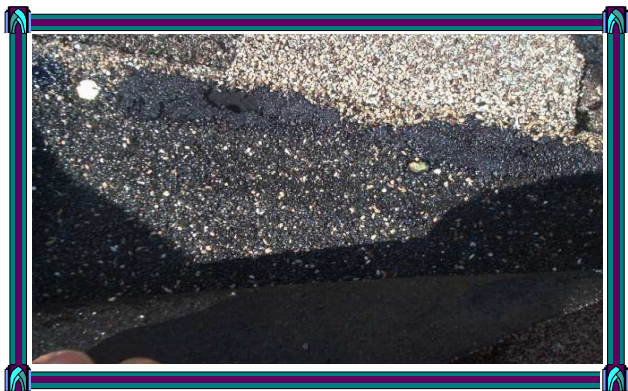
Another overdriven nail in the field of the roof.
