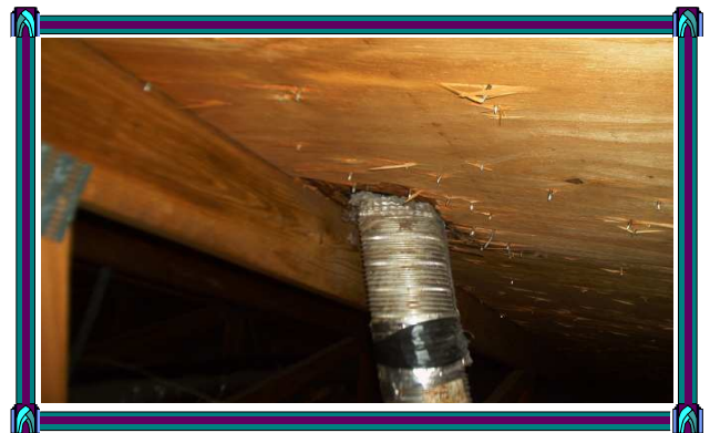
Rotted/damaged wood at bathroom vent fan vent stack.
