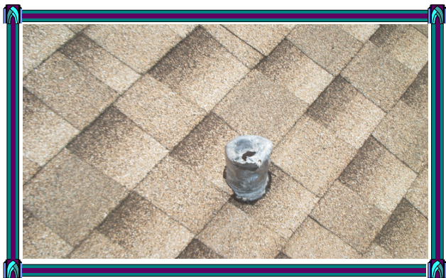
Another vent stack not changed.
