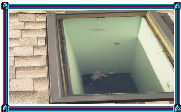
Tar on skylight.
