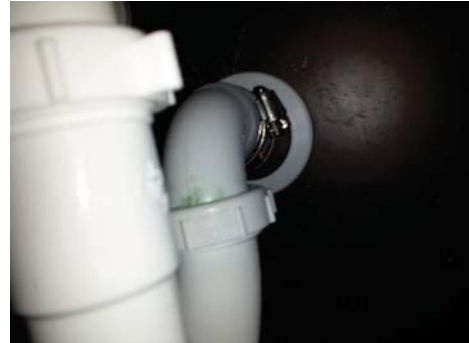
Improper drain line connection observed at right side master bathroom sink.
