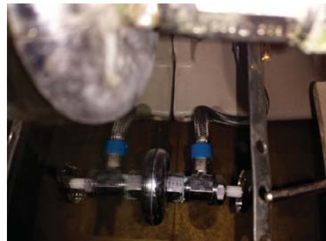
Drain stopper rod was disconnected at hall bathroom sink.
