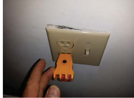
Receptacles at master bedroom and at kitchen were not secured to boxes properly.
