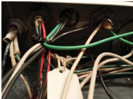
Improperly secured conduit observed at top of breaker panel.
