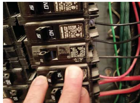
Several different manufacturers of breakers were used in this panel.
