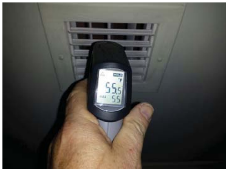
Cooling cycle being tested.
