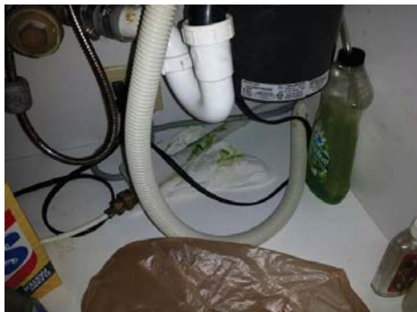
There was no high loop present at the dishwasher drain line which may allow waste water to back flow into the dishwasher.
