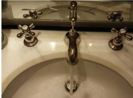
Both fixtures were loose as right side master bathroom sink.
