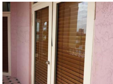
Several exterior doors did not close properly or required some sort of adjustment and had damaged seals.
