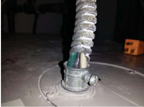
Improper connection observed at water heater.
