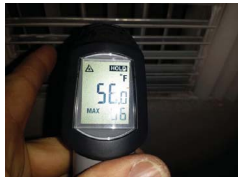
Cooling cycle being tested.
