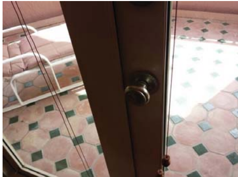
Numerous primary and secondary door locks did not function.
