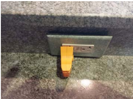
Receptacles at master bedroom and at kitchen were not secured to boxes properly.
