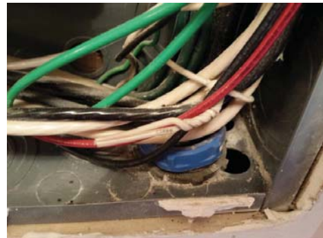
Void observed at bottom of breaker panel.
