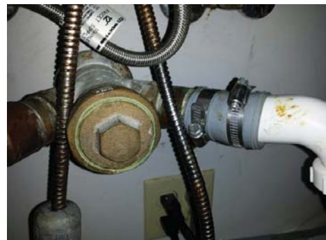
Improper connection at right side kitchen sink drain line.
