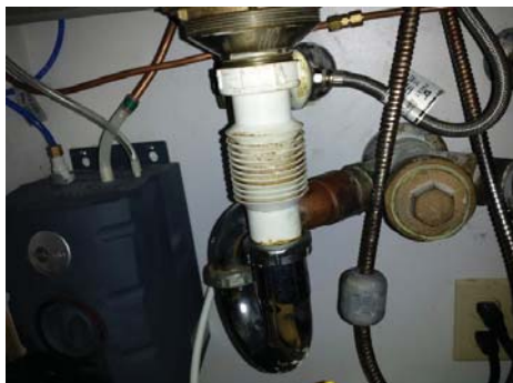
Improper drain line (rigid is required) at kitchen sink.
