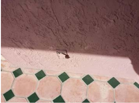
Several exterior receptacle covers were broken at the balcony.
