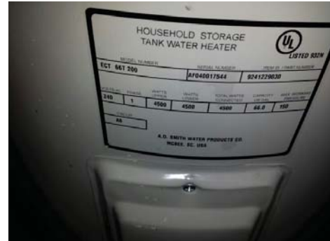
Water heater data plate.
