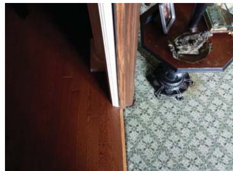
Pocket door at left side of unit did not function.
